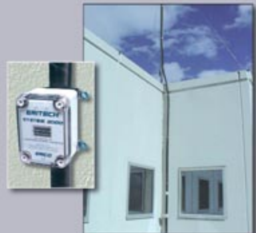
The ERITECH System 3000 ERICORE downconductor is easily retro-fitted to existing structures. Inset: ERITECH Lightning Event Counter (LEC IV) installed to register strikes to System 3000.
